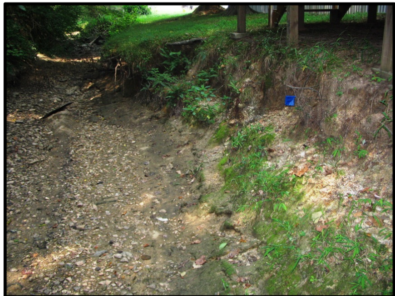
Eroded stream bank adjacent to existing residence
