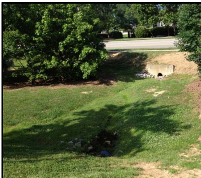
Existing depression between Louis Stephens Road and parking lot
