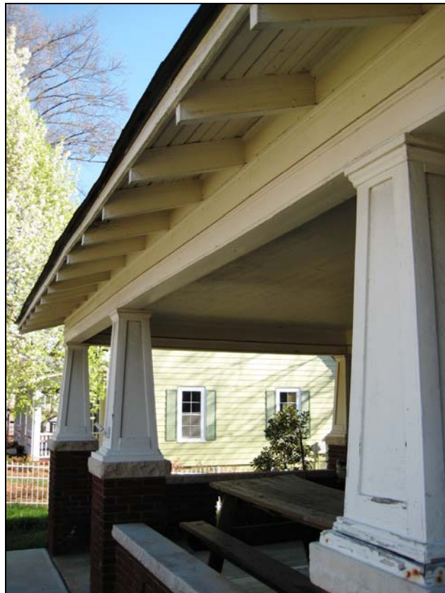
Exposed Rafter Ends
