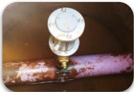
Air Release Manholes & Valves 65
