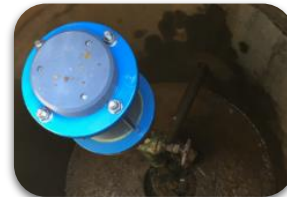
Air Release Manholes & Valves 825
