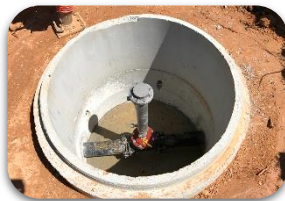
Air Release Manholes & Valves 175
