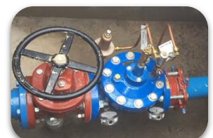
Control Valves 9 Locations
