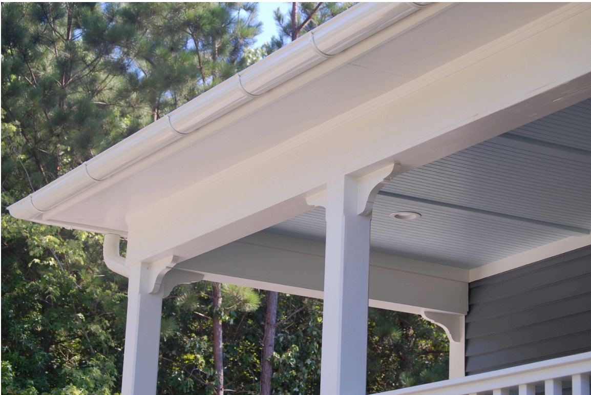
John L. and Henrie G. Sears House, porch posts and brackets, viewNE
