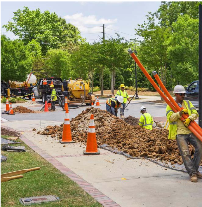
Access to fiber-optic cable networks is growing throughout Cary.
