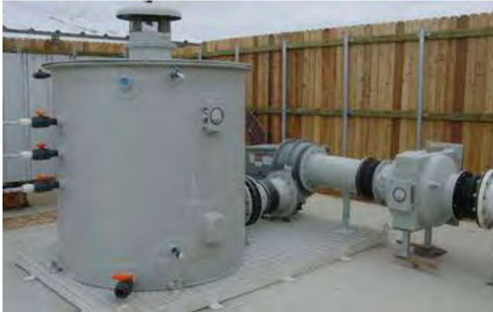
Figure 3-6: Carbon Odor Scrubber
