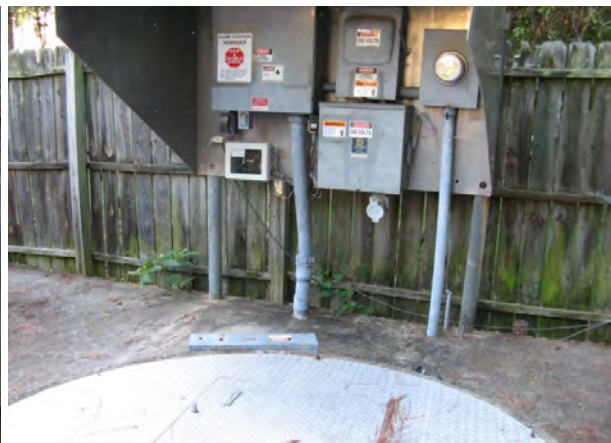
Control Panel & Wetwell
