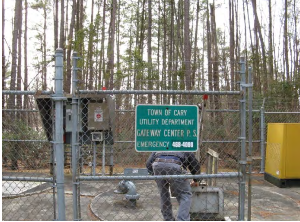
Gateway Center Pump Station
