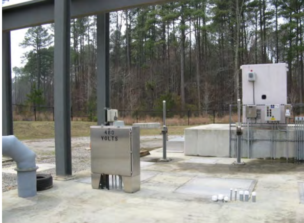
Morris Branch Pump Station
