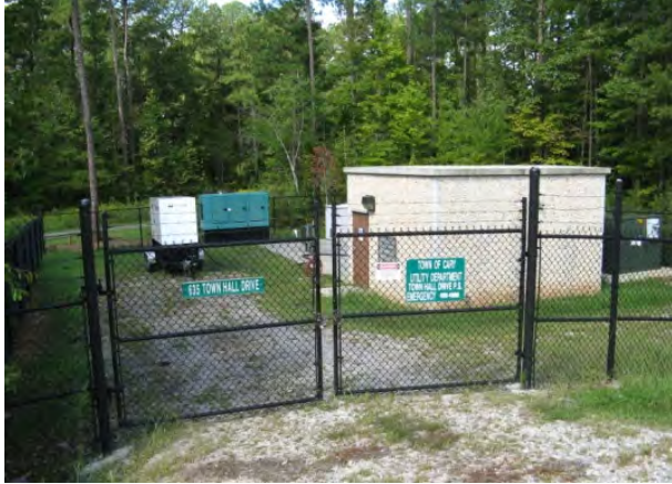
Town Hall Dr Pump Station
