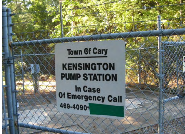
Kensington Pump Station
