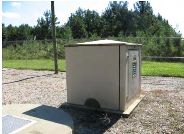
Grinder Hydraulic Unit
