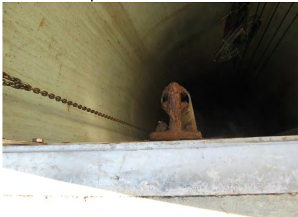
Rust on Pump Guide Bracket
