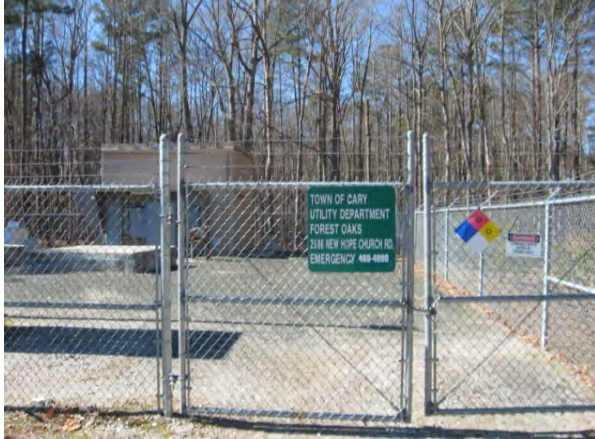
Forest Oaks Pump Station
