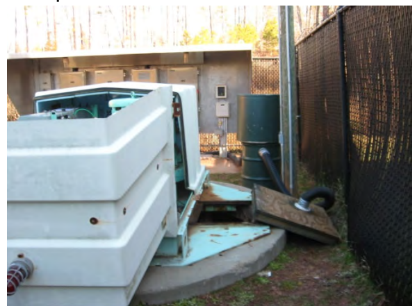
Pumps Enclosure & Odor Control
