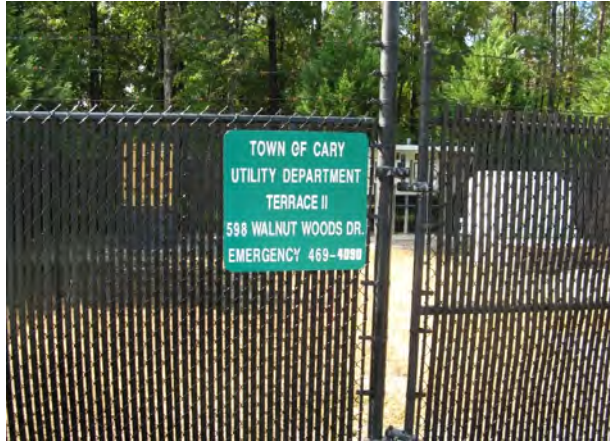
Terrance II Pump Station
