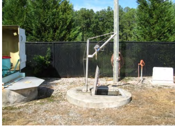
Tash Rack Crane
