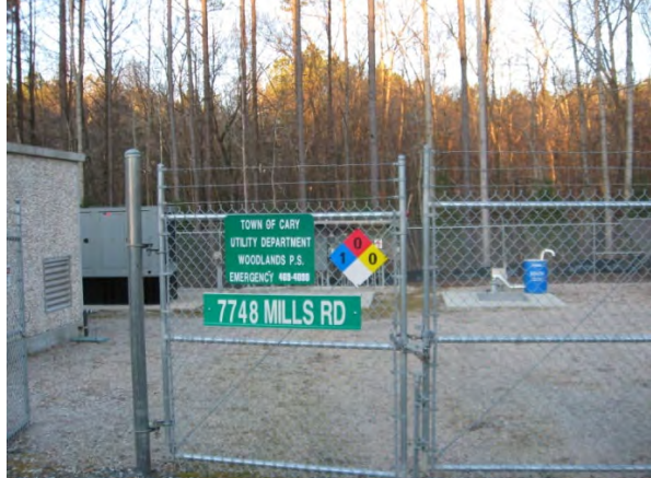
Woodlands Pump Station
