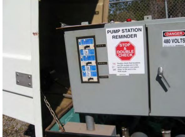
Pump Control Panel
