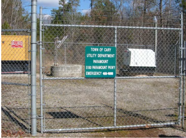
Paramount Pump Station
