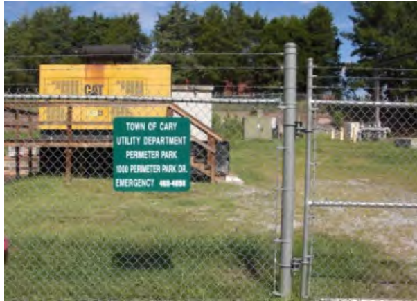
Perimeter Park Pump Station
