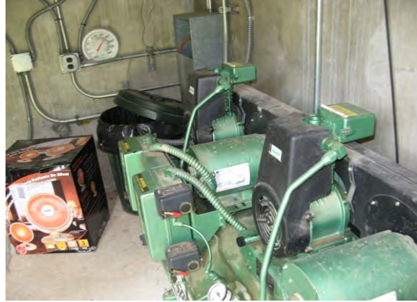
Compressor for Bubbler System
