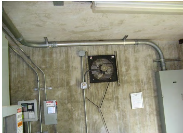
Electical Room Exhaust Fan
