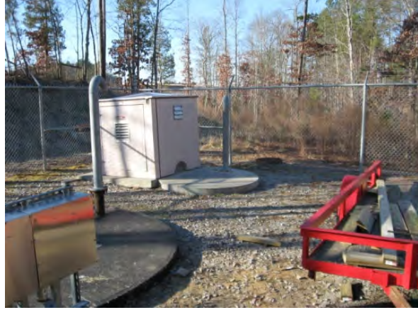
Kitts Creek Pump Station
