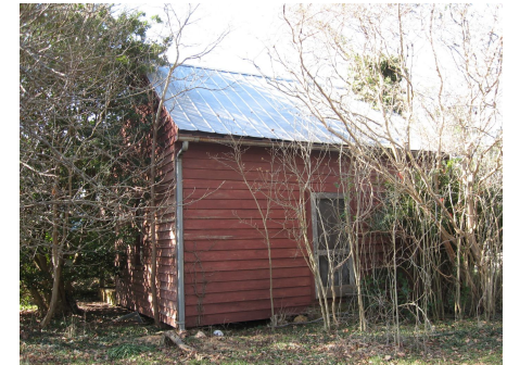
Above two pictures: The Bartley farmhouse (ca. 1840s) and outbuilding on Penny Road are part of a 50-acre property acquired by the Town of Cary for a future community park.
