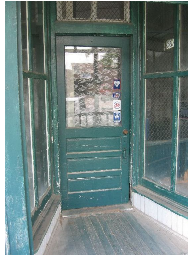
In Carpenter, the Ferrell Store's entrance retains original display windows, flooring, and single-light, three-panel wood door.
