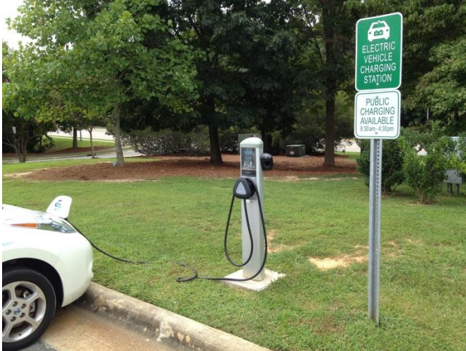
Electric Vehicle Charging Station at the Garmon Operations Center
