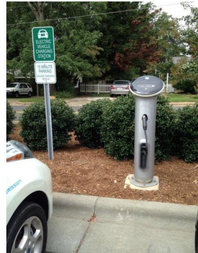
Electric Vehicle Charging Station at the Cary Art Center
